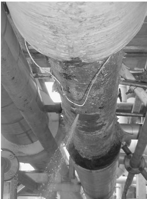
1.2 Examples of CUI damage to carbon steel piping and equipment.
